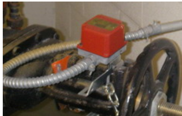
Tamper switch on a sprinkler valve
